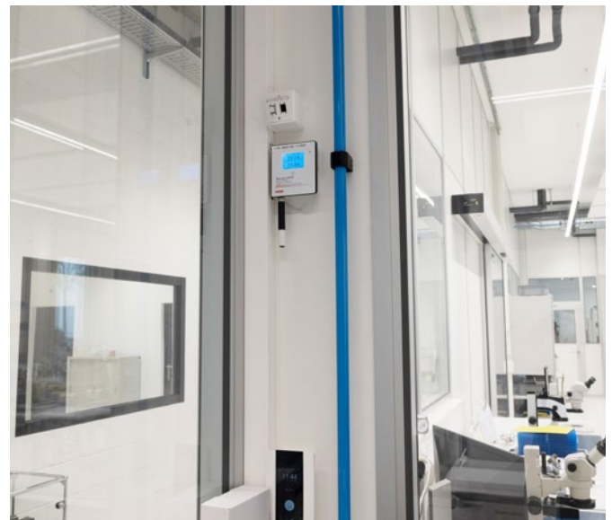
The measured values, in this case, temperature and humidity, can be checked at any time both on the individual data loggers and on the dashboard on the computer.
