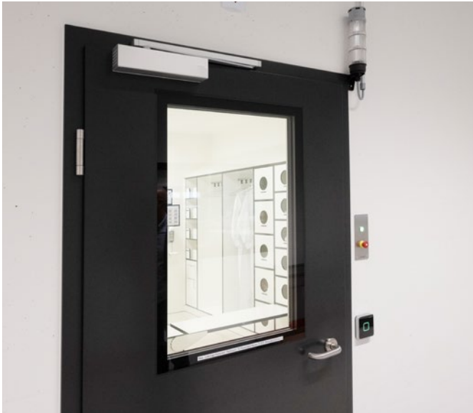
View of the personnel airlock in the new cleanroom. An RMS indicator light has been installed above the door, which triggers an audible and visual alarm in an emergency.
